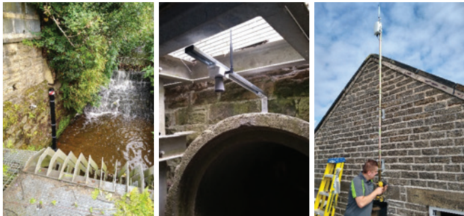
FloodAlert sensors and LoWaRAN® network gateway installation at Crimble Clough, Slaithwaite
